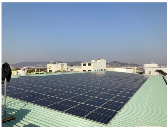
【Solar panels installed at rooftop of Itami Plant】
